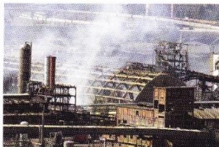
Nitrates can decompose explosively to cause a large amount of damage, as shown by the remains of this fertiliser factory.
